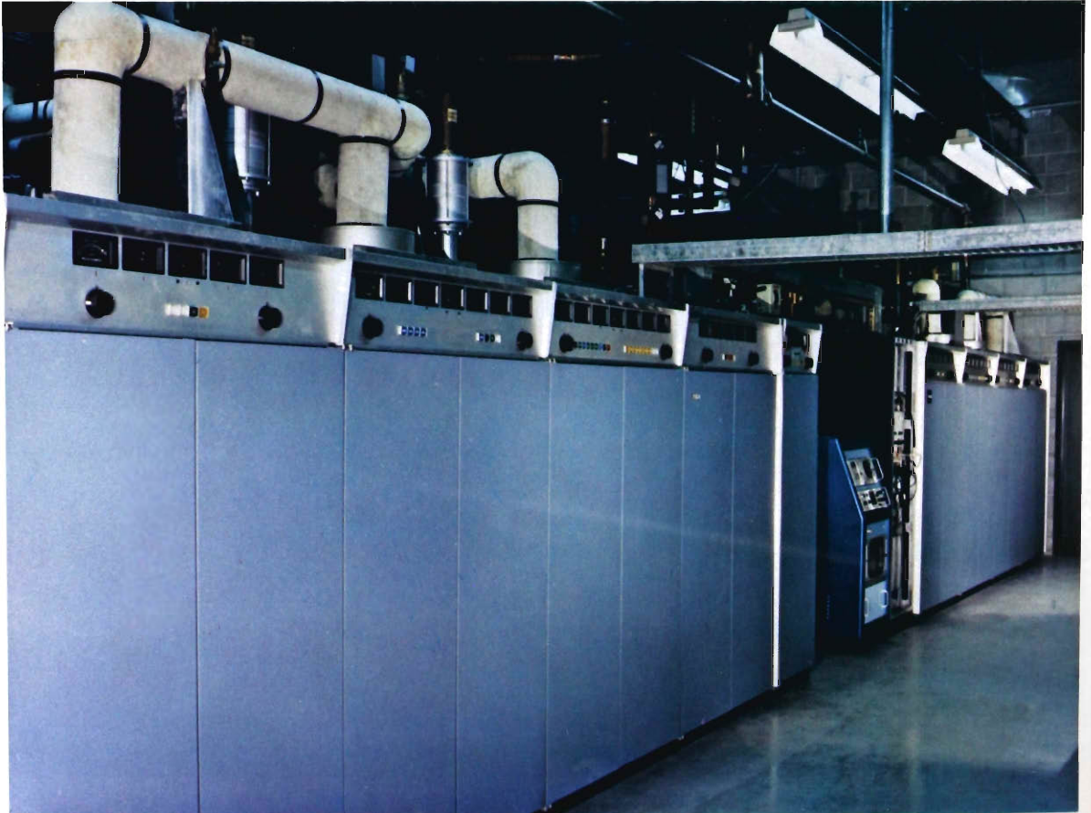
1. Parallel transmitter installation at WKBG-TV, Boston.
