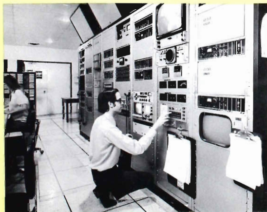
Remote controls for transmitter and microwave system are rack-mounted behind camera control position of console.
